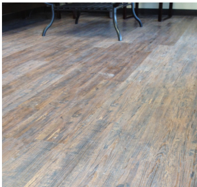
Worn LVT Floor
